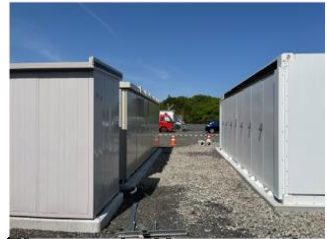
Storage batteries and cubicles
